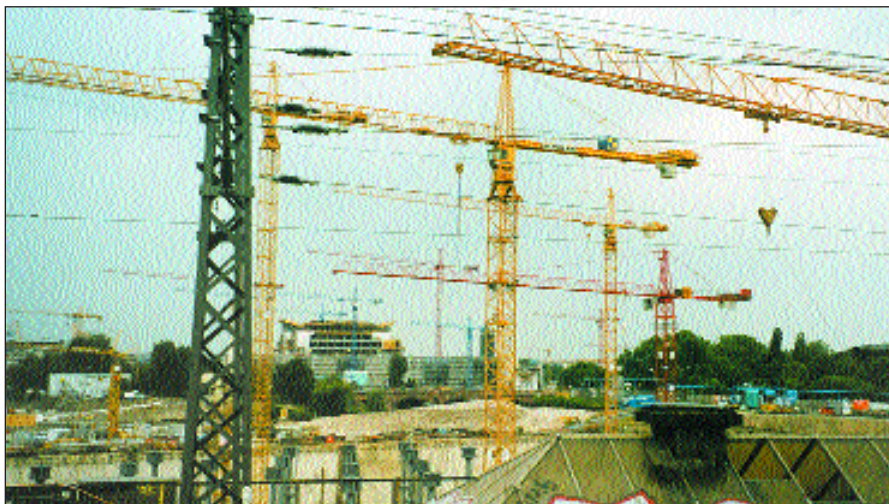
Dozens of construction cranes towering over the site of Berlin's new railway depot symbolize the emerging strength of a reunited Germany, Europe's economic powerhouse.
