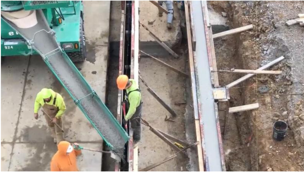
Concrete is being poured for a new retaining wall alongside the existing warehouse loading dock.
